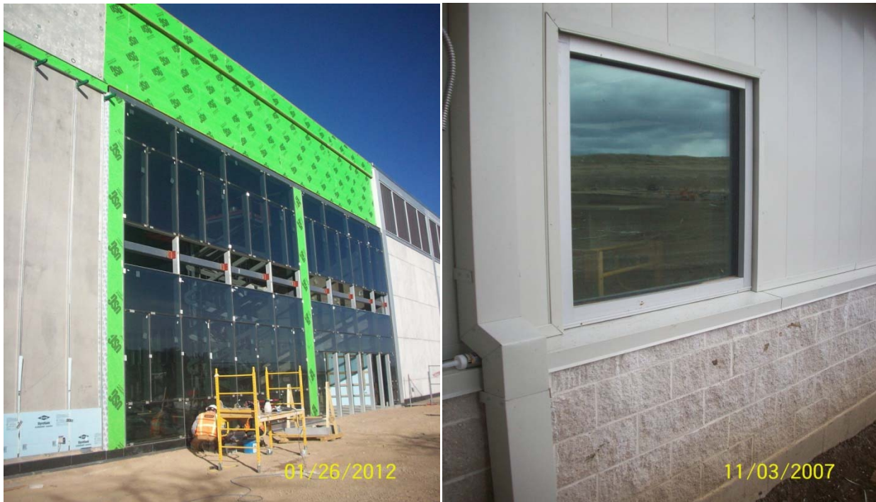
Figure 2: (Left) is an example of a large curtain wall assembly commonly seen in construction applications. (Right) a small fixed aluminum frame window.
