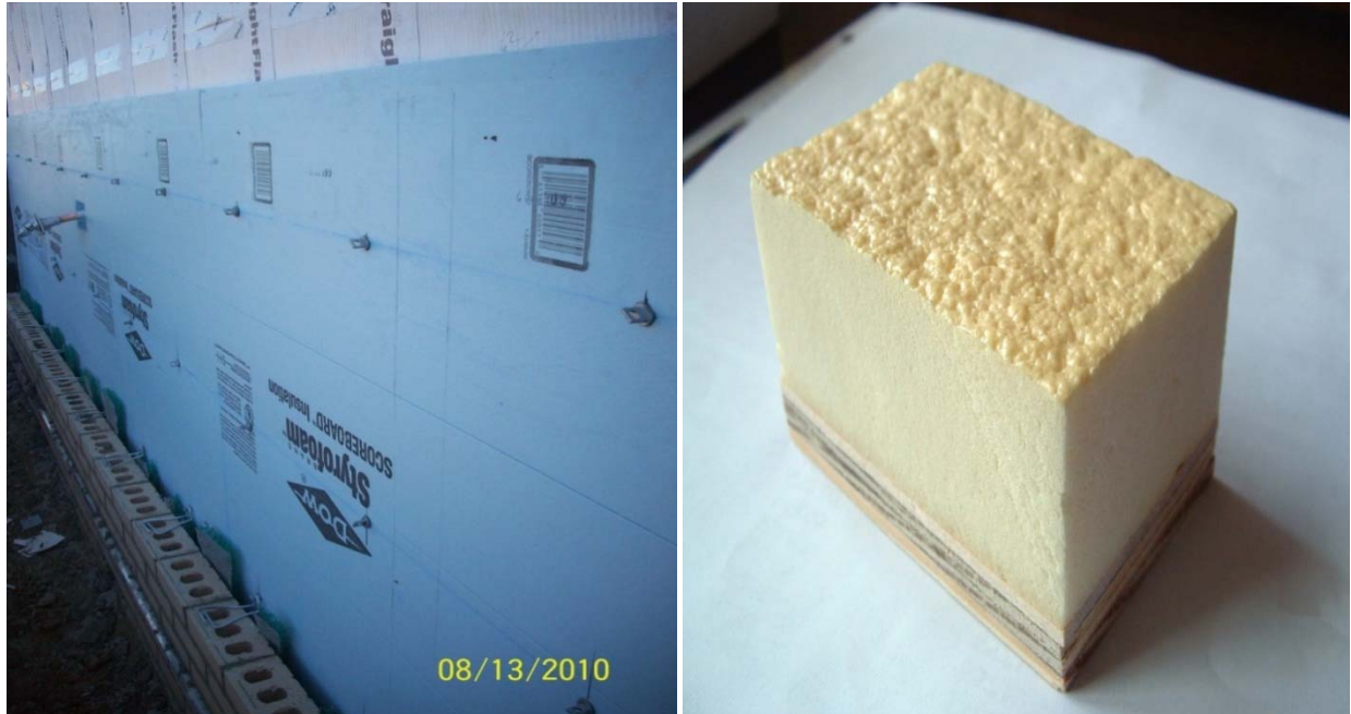
Figure 4: (Left) This installation of the exterior insulation board in this figure is of high quality. Note the boards and joints between them are tight with no large gaps present. Brick ties shown in this installation to are not interfering with the continuity of the insulation and are actually designed to double as fasteners for the insulation boards to the substrate. (Right) An example of a closed cell spray foam insulation material.
